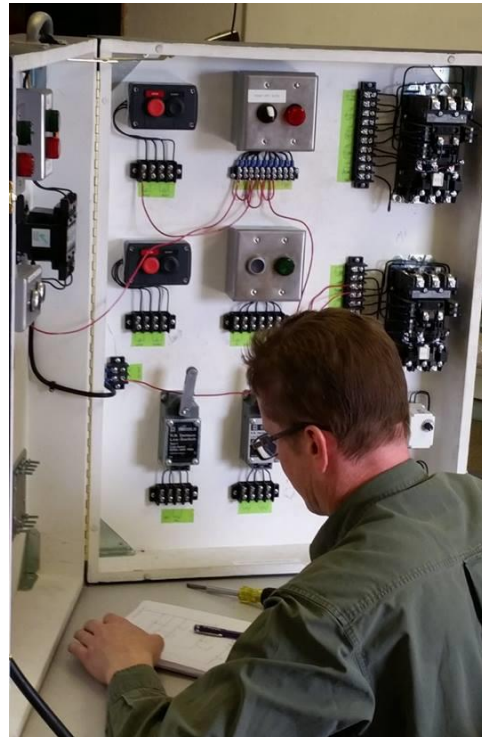
Apprentice David Wallis working on the motor control installation part of the competition.
